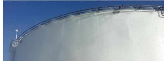
Figure 2: Fire water cooling system in operation
