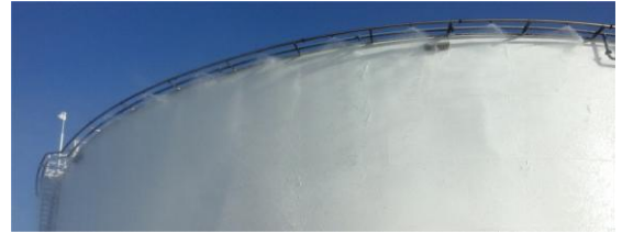
Figure 2: Fire water cooling system in operation
